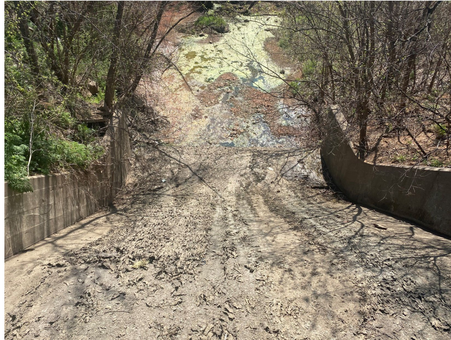
Downstream of the pond with extreme signs of stream degradation
